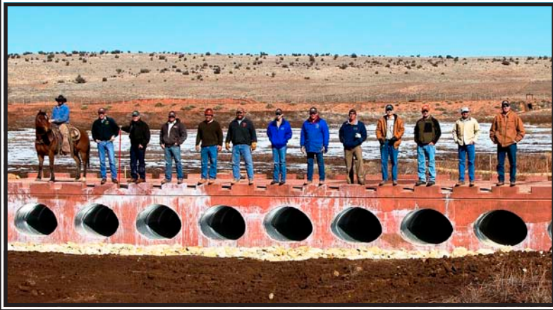
Redlands Crossing is a concrete bridge made up of an array of culverts, designed to move water during flash floods.
